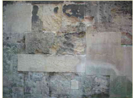
Figure 19. Weathering and repairs on the stretch of wall between the Danby Gateway and the Library and Herbarium
