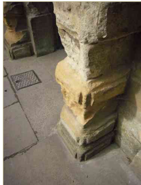
Figure 13. Damage to Headington freestone on the eastern gateway
