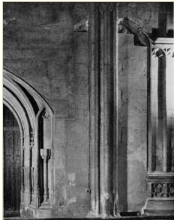
Figure 6. East door of Divinity School with exposed blocked window and original panelling behind, exposed during restoration work in the 1960s
